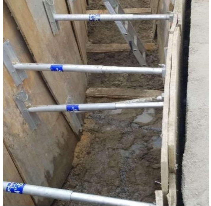
Fig 2: Groundwater seeping into trench along Colovos Rd. Viewing north. (6-27-19).
