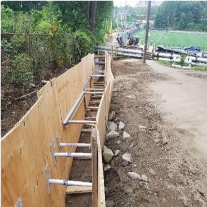
Fig 5: Excavating trench next to field house, working towards steam pipe. Viewing south. (6-27-19).
