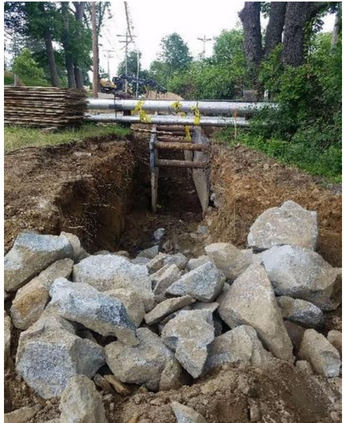
Fig 4: Excavating for trench under the steam pipe next to field house. Viewing north. (6-27-19).
