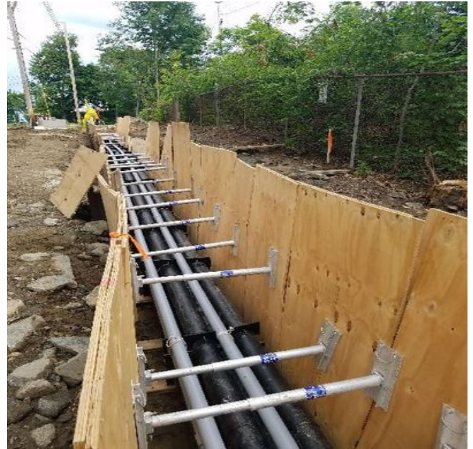
Fig 18: McCourt continues to install pipe in trench next to field house. Viewing north. (7-02-19).
