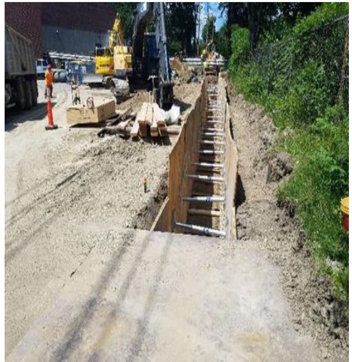
Fig 12: McCourt trenching next to field house, heading towards steam pipe. Viewing north. (6-28-19).
