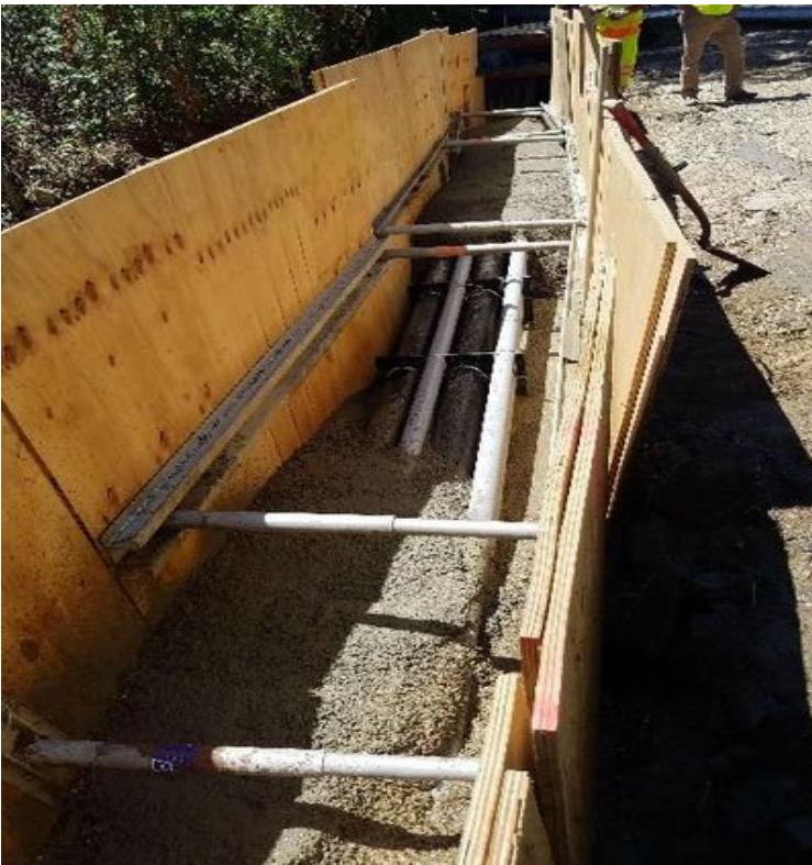
Fig 19: Pouring concrete duct bank in trench next to field house. Viewing south. (7-02-19).
