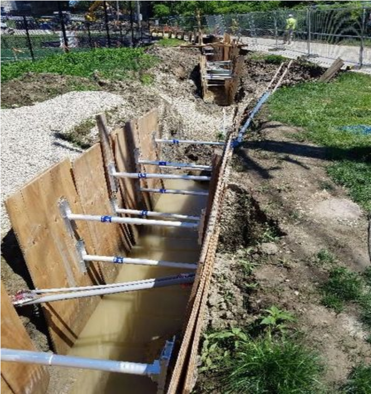
Fig 13: Water collecting in trench along Colovos Rd. Viewing north. (7-01-19).
