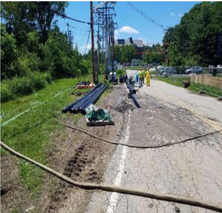
Fig 15: McCourt cont. to fuse pipe to install in trench along Colovos Rd. Viewing south. (7-01-19).
