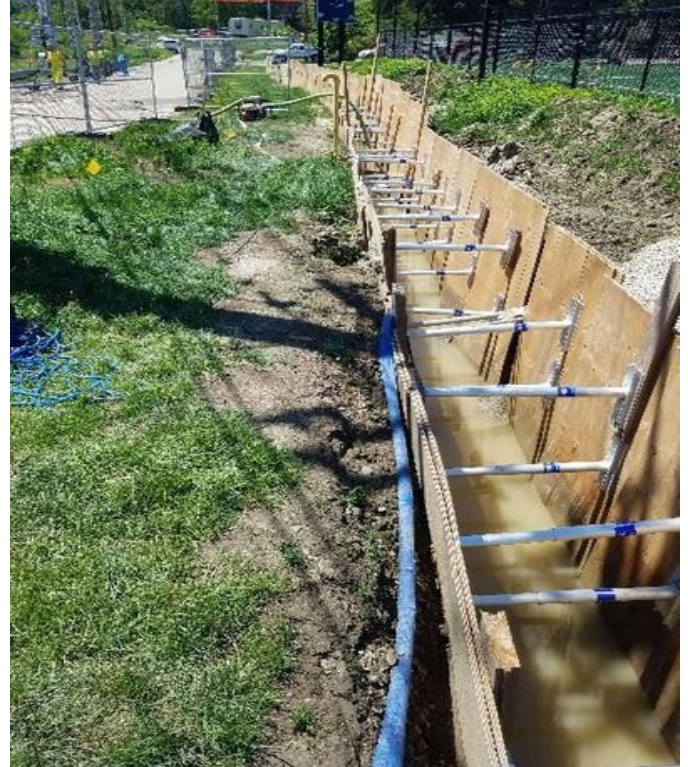
Fig 14: McCourt continues to pump water out of trench along Colovos Rd. Viewing north. (7-01-19).
