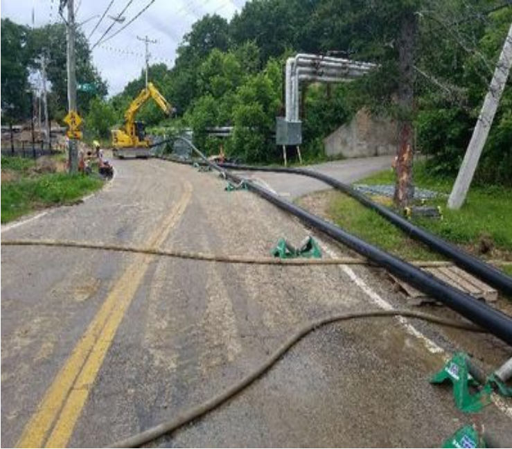
Fig 17: McCourt fusing and installing pipe in trench along Colovos Rd. Viewing north. (7-02-19).
