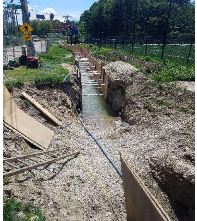
Fig 10: Water collecting in trench along Colovos Rd. Viewing south. (6-28-19).
